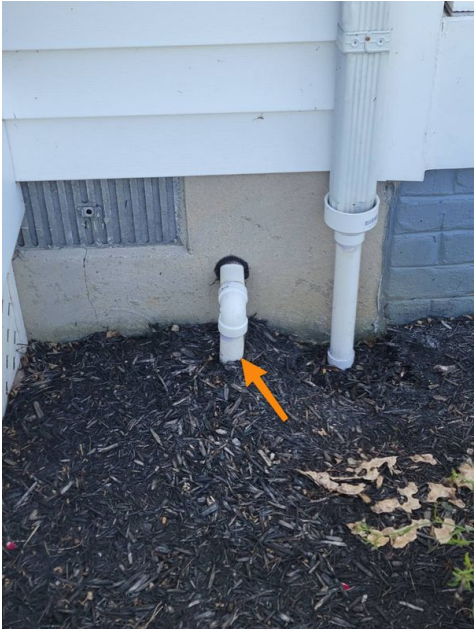
Discharge Below Grade Limits Inspection
