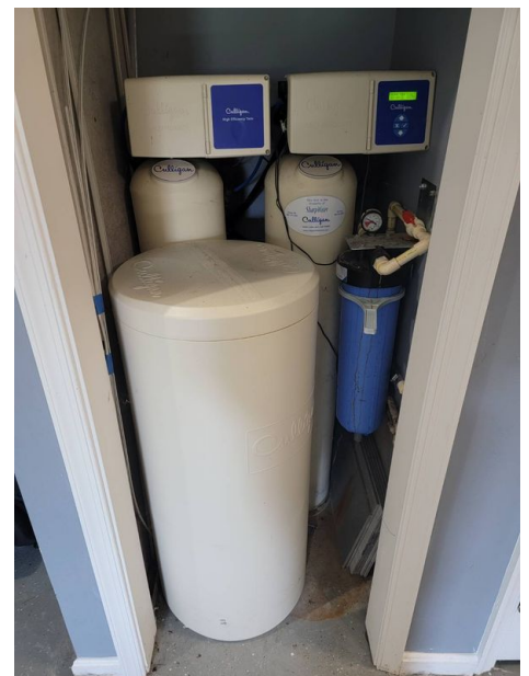
Water Conditioning System (Visually inspected only)
