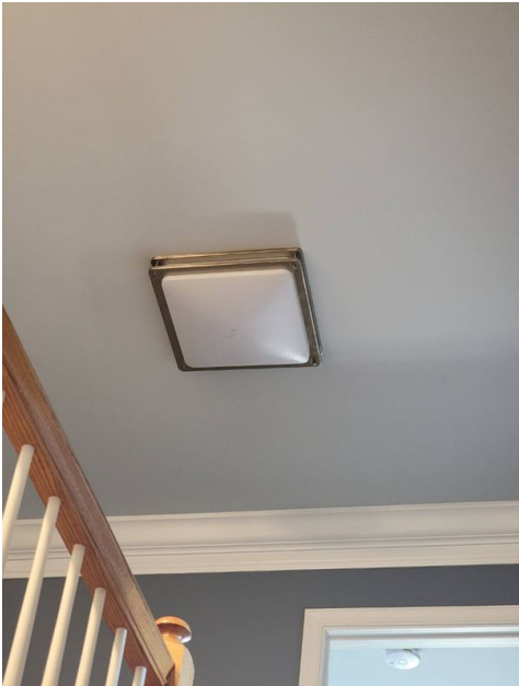
Inoperative Light Fixture (Upstairs Hallway)
