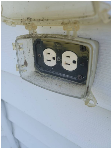
No GFCI Electrical Protection
