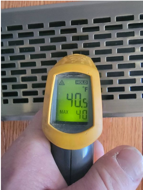
Supply Temperature (Cooling)See Comments
