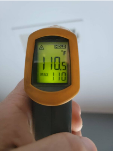
Electric Back-up Heaters Functional
