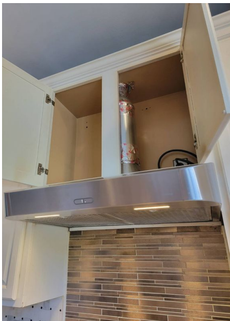
Ventilation Overhead External Discharge
