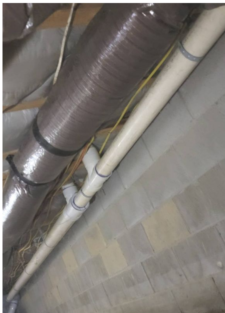
Drain Waste Pipes PVC Pitched Properly
