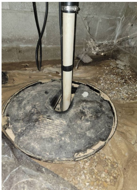
Sump Pump Functional (Lifted Float)
