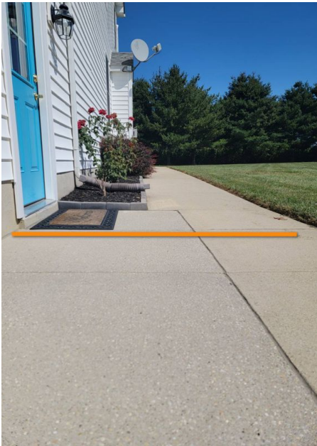
Grading(Right Side) Neutral -See Comments
