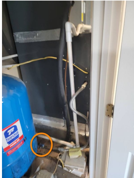
Furnace Gas Shut-off Valve Utility Closet Garage
