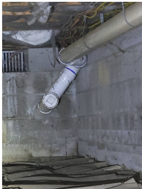
Clean-out (Septic/Leaving Right Side of Crawl Space)
