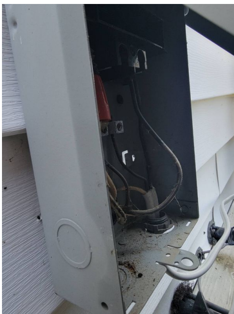
Missing Cover Plate (Leaving Exposed Wiring Accessible)
