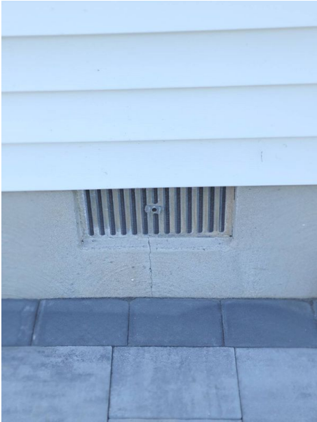
Manual Crawl Space Vents (See How to operate)
