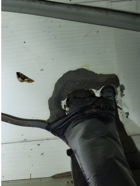
Gaps needs Sealing
