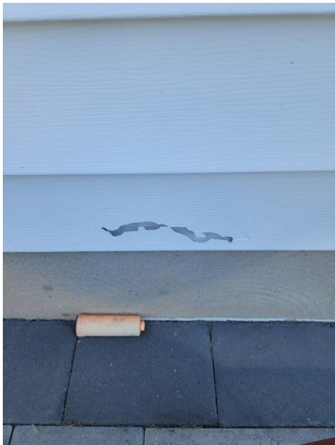
Damaged Vinyl Siding
