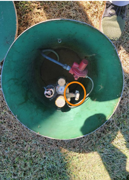
Underground Propane Tank and Main Shut-off Valve
