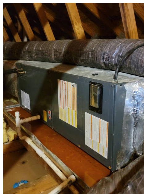
Attic Air Handler for Heat Pump (See Comments)
