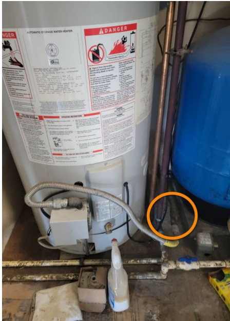
Water Heater Gas Shut-off Valve Utility Closet Garage
