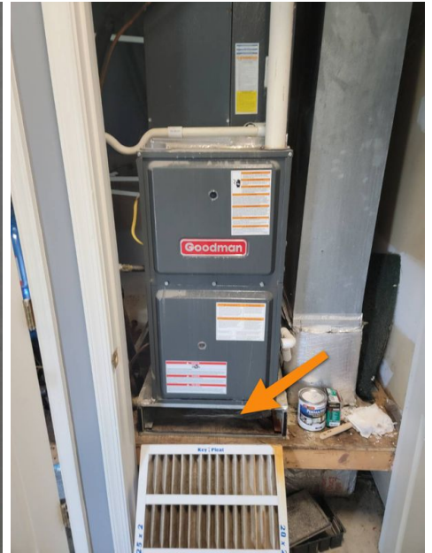
High Efficiency Furnace (Propane) Filter Location
