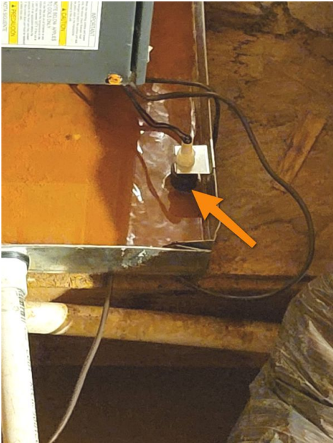
Water Safety Device not Functioning
