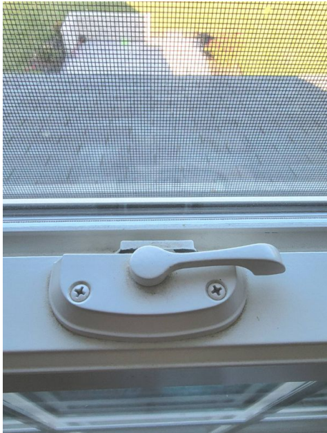
Latch doesn't line up to latch properly
