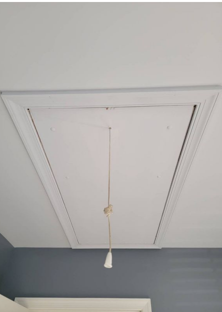
Attic Access Pull Down Steps
