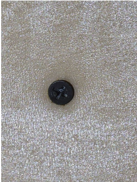
Drywall Screws Securing Cabinets
