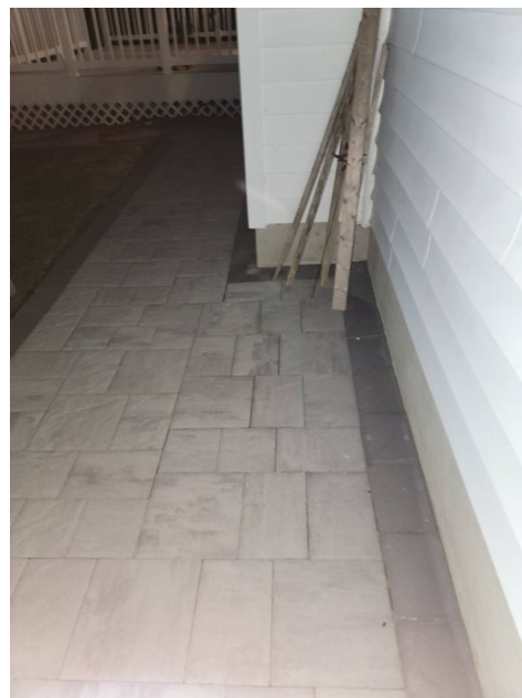
Rear Slots between pavers are allowing Water to pass through foundation
