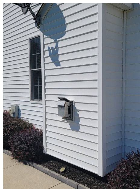
Fireplace Direct Vent in Framed Enclosure
