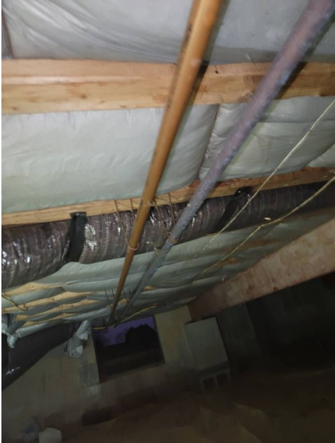
Under Floor Insulation installed Backwards
