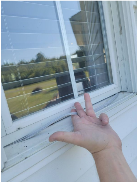
Weather Seal Shifted out of place
