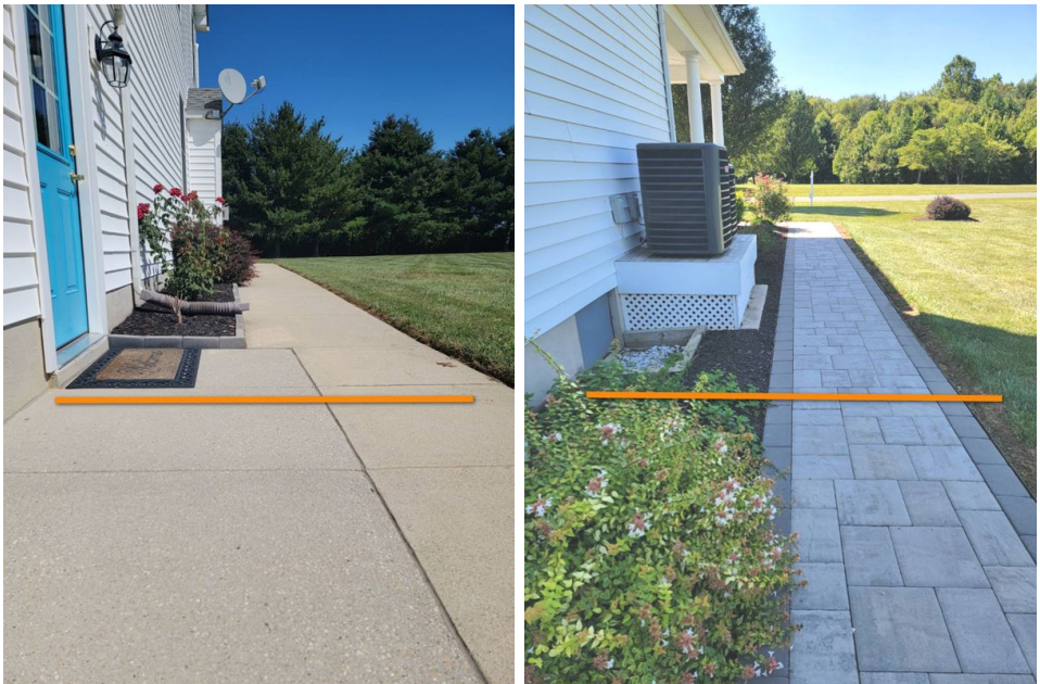
Neutral Grading no positive slope away from Foundation
