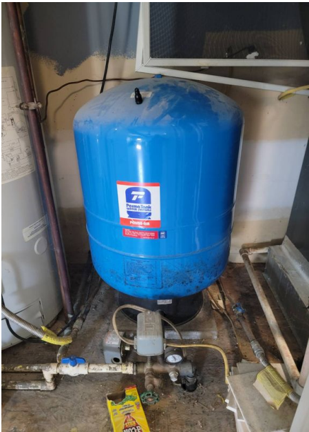
Pressure Tank Functional
