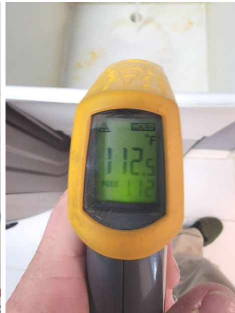
Hot Water Temperature Acceptable
