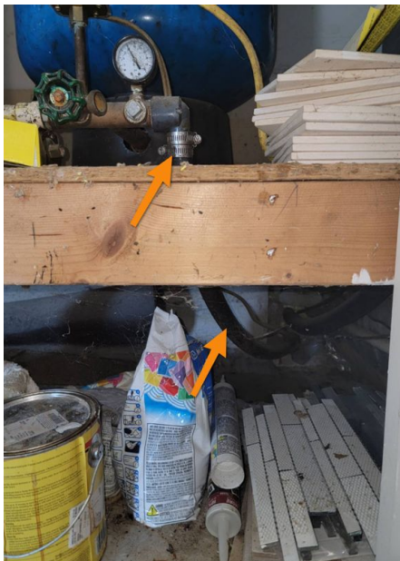
Incoming Water Line HDPE High Density Polyethylene
