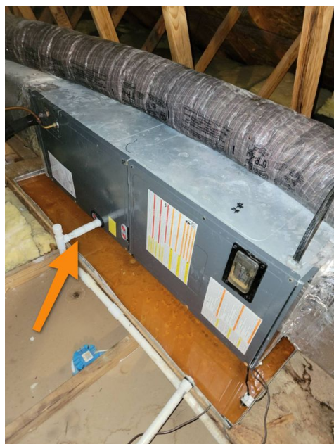
Drain needs clearing here
