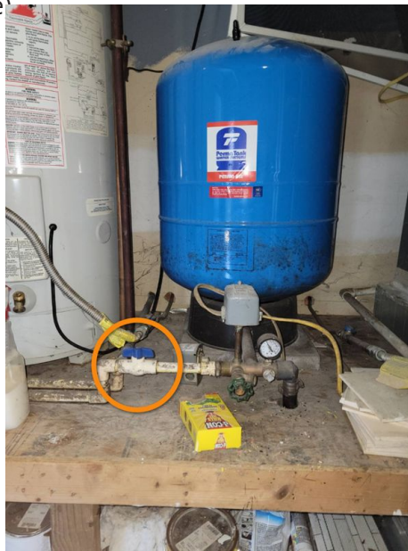
Main Water Shut-off Valve Utility Closet/Garage
