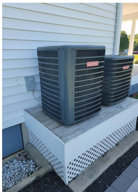
Heat Pump (Left Side Unit) See Comments
