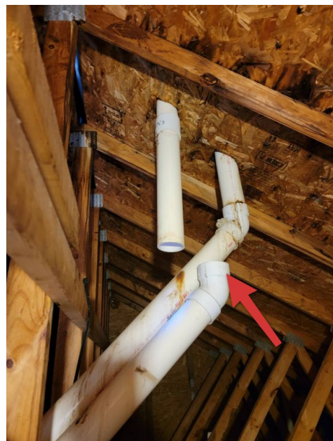
Must Be Reconnected before using the furnace downstairs
