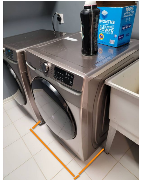
Missing Water Catch Pan
