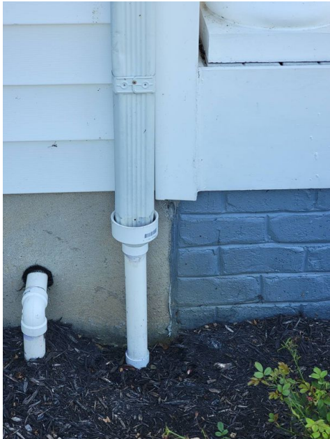
Downspout discharges below grade limits inspection
