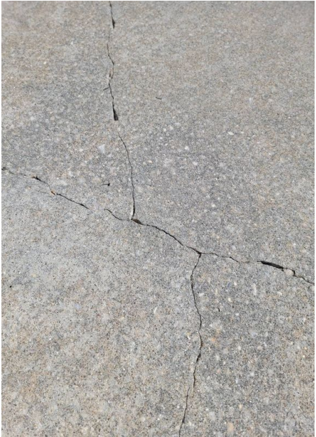
Minor Cracking (Maintenance)
