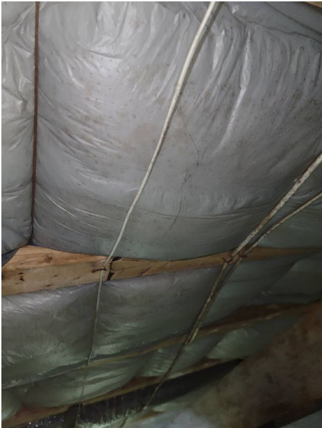
Under Floor Insulation Fiberglass Batts (See Comments)
