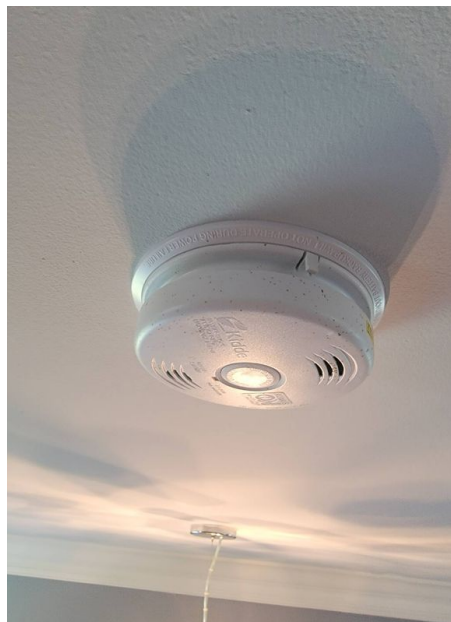
Smoke and Carbon Monoxide Detectors Acceptable
