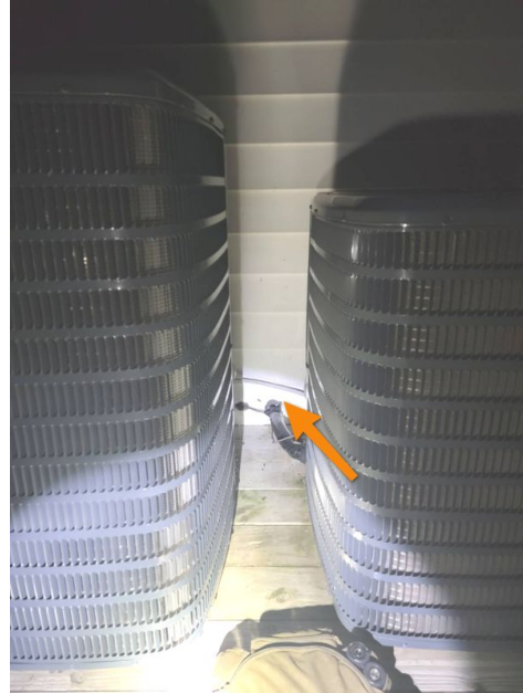
Wall Between both HVAC outdoor units
