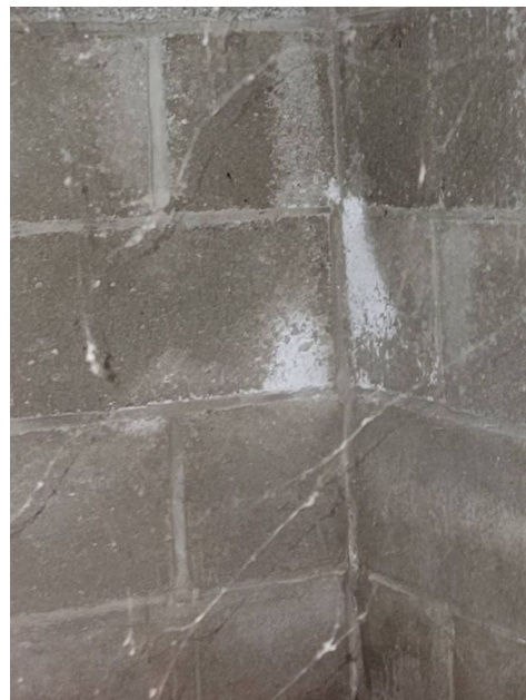
Efflorescence White Powder Calcium Carbonate
