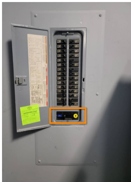
Main Electrical Shut-off Switch (Garage)
