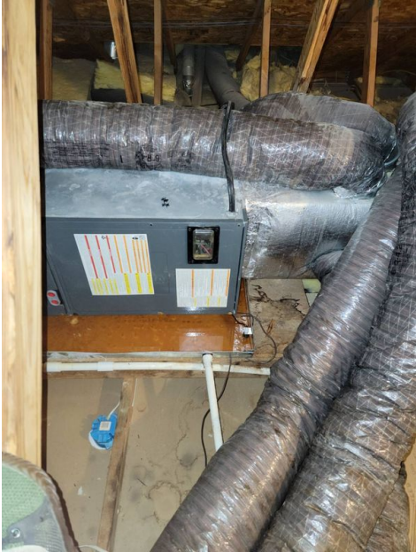
Metal and Flex Ductwork
