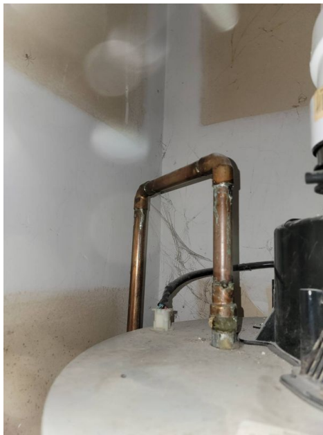
Copper Water Distribution Lines
