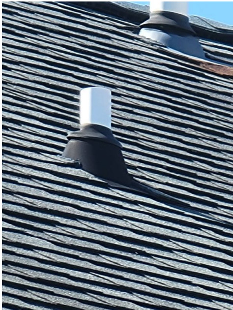
Vent Pipes too short
