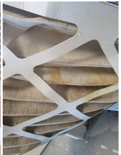
Water Staining on Filter indicates (Coil Freezing/Melting)
