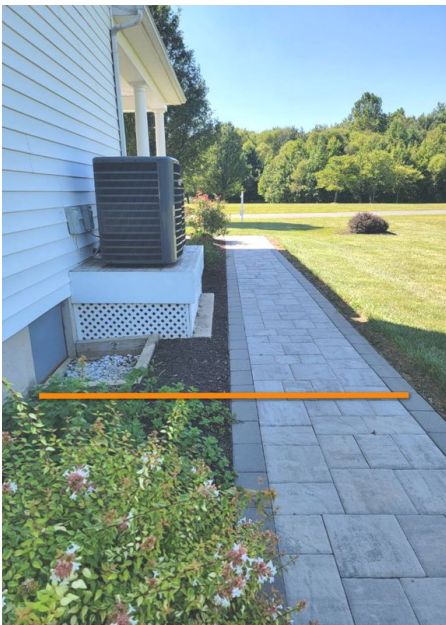
Grading(Left Side) Neutral -No positive slope away from Foundation
