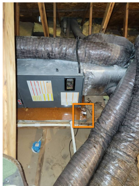
Water Cut-off switch not working to shut off system properly
