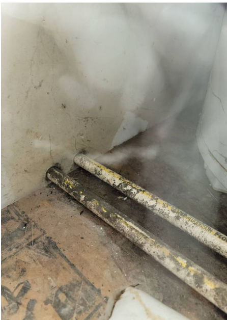
CPVC Water Distribution Lines
