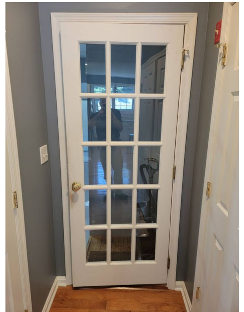
Garage Occupant Door not Fire Rated
