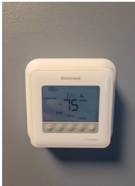
Upstairs Hallway Thermostat Functional
