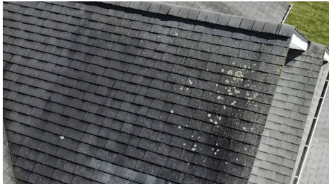
Biological Growth Needs Cleaning
