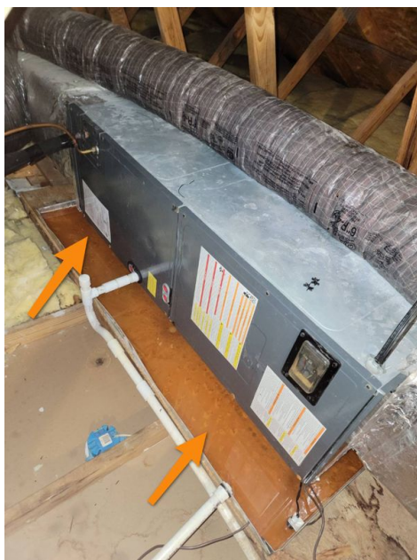
An inch of standing water in catch pan
